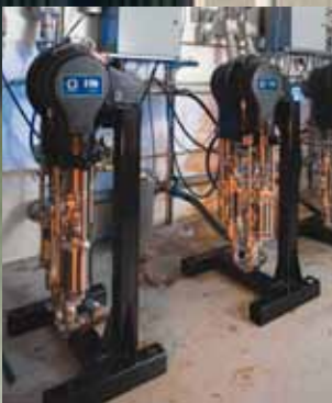
Setup of a modern paint kitchen
